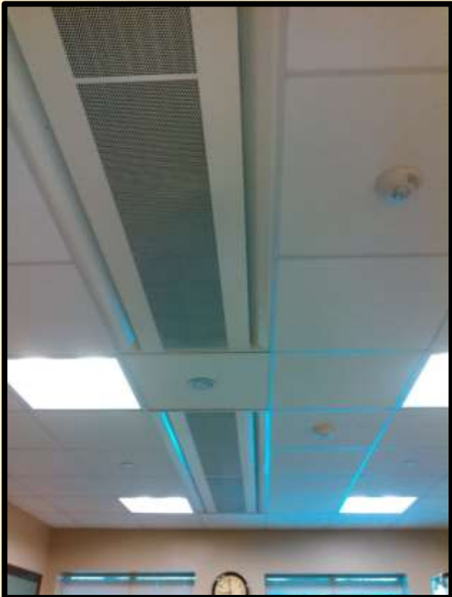
Chilled Beam at Franklin Library
