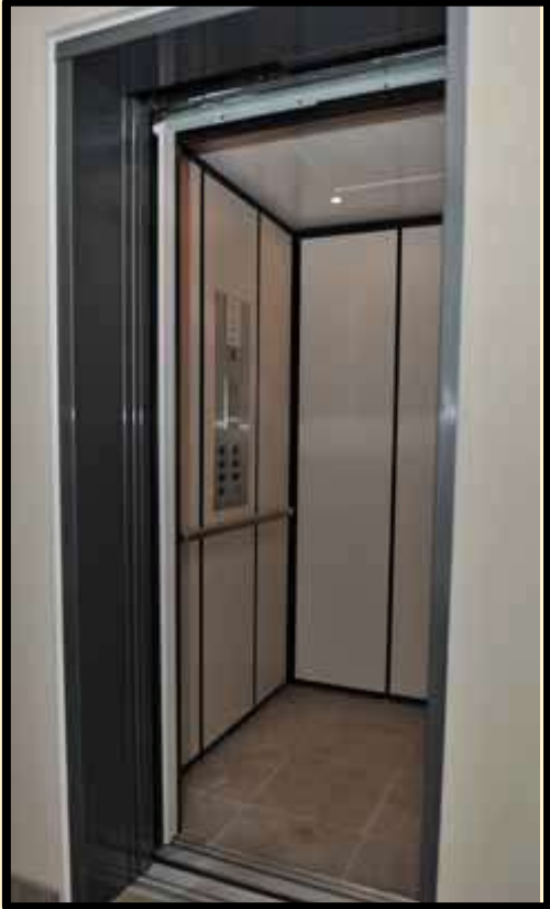
Example of Elevator Cab
