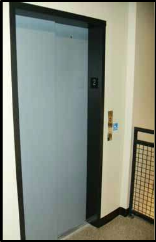
Example of Elevator Door
