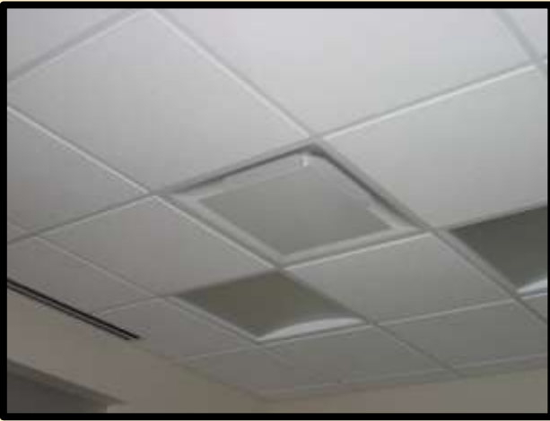
Fan Coil Units and VAV Units in the City Manager's Office
