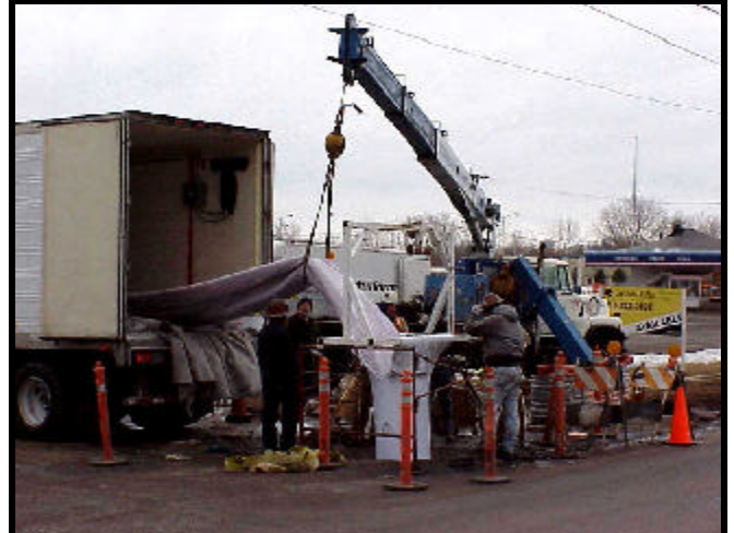
The flexible liner is placed into the sewer then water is pumped into the liner, forcing the liner to take the shape of the pipe. The water is then heated with a boiler system so as to set the resin, creating a hard shell inside the sewer pipe.
