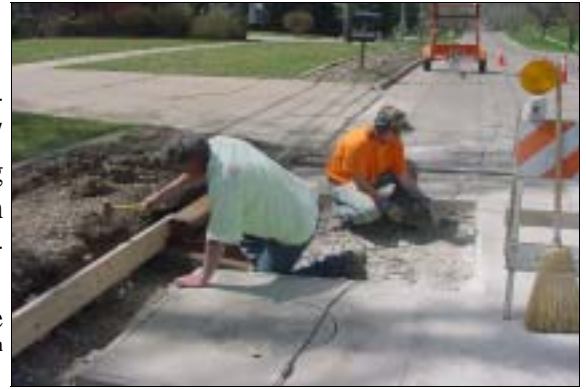
Sewer Maintenance Worker Dennis Dearth sets forms as Bradley Sage drills to install rebar.
